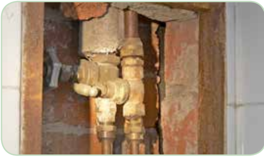
Friable asbestos lagging on pipes
