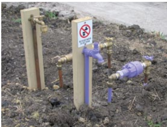
Recycled water and drinking water meter assemblies
