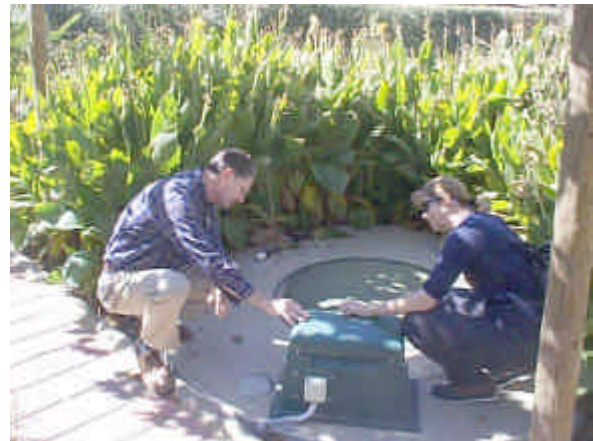
An established AWTS integrated with the landscape. The background flora thrives on the treated effluent that is reused via subsoil irrigation.
