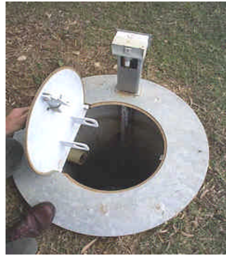
An example of an easy lockable access ground level lid to AWTS.
