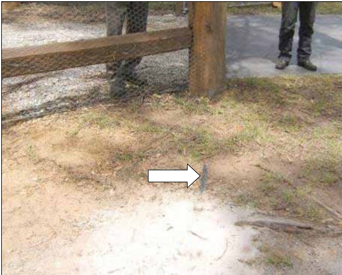
Figure 2.2 Main irrigation line buried at only 50 mm under gravel driveway – 500 mm is the minimum required depth.
