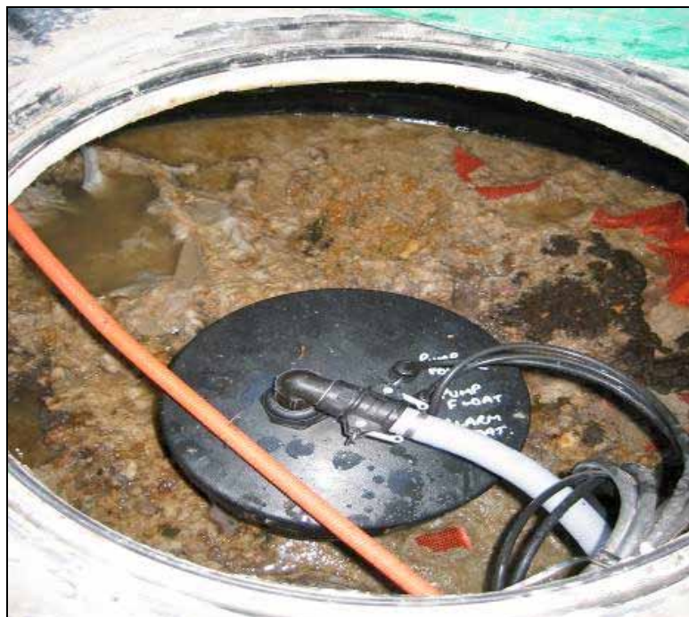
Figure 5.10 A flooded system due to pump failure
