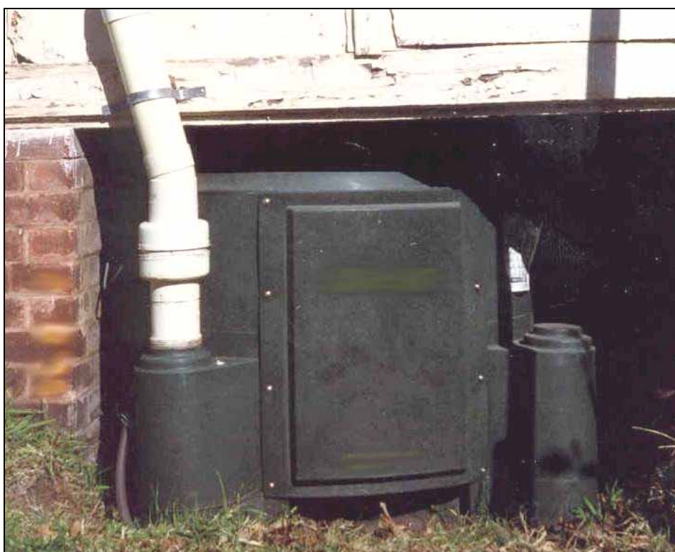
Figure 6.1 A composting unit used in conjunction with a composting toilet
