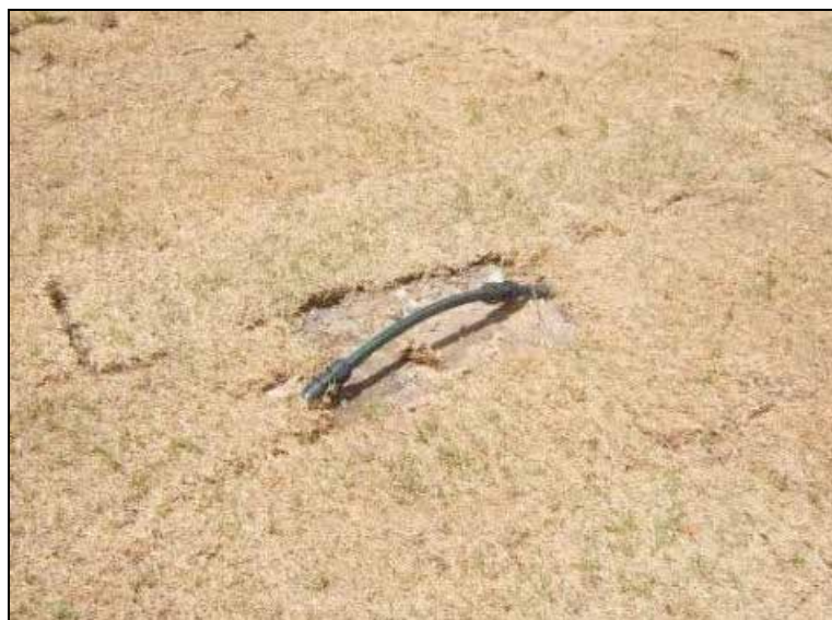
Figure 13.8 Damaged irrigation line sections cut out and replaced as part of an unsatisfactory repair.
