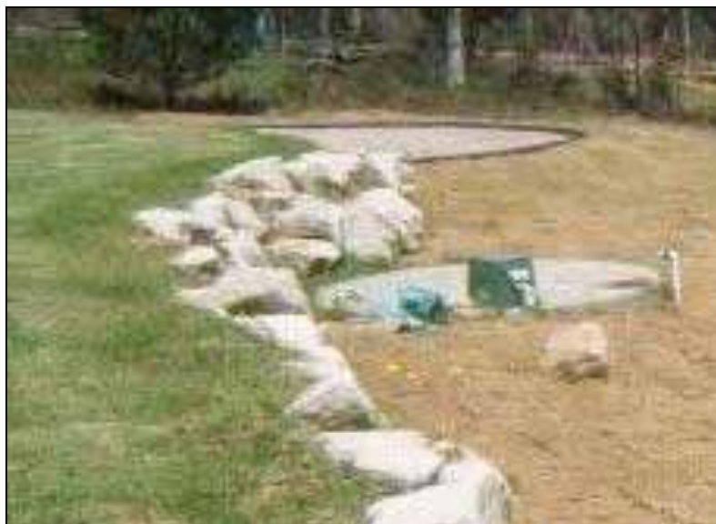
Figure 13.10 One of the new fields at the rear of the property established upslope of the aerated wastewater treatment system on imported soil
