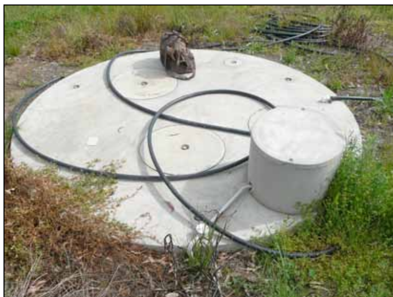
Figure 4.9 New AWTS with irrigation hose coiled on top, no sprinklers and potential for stormwater inundation
