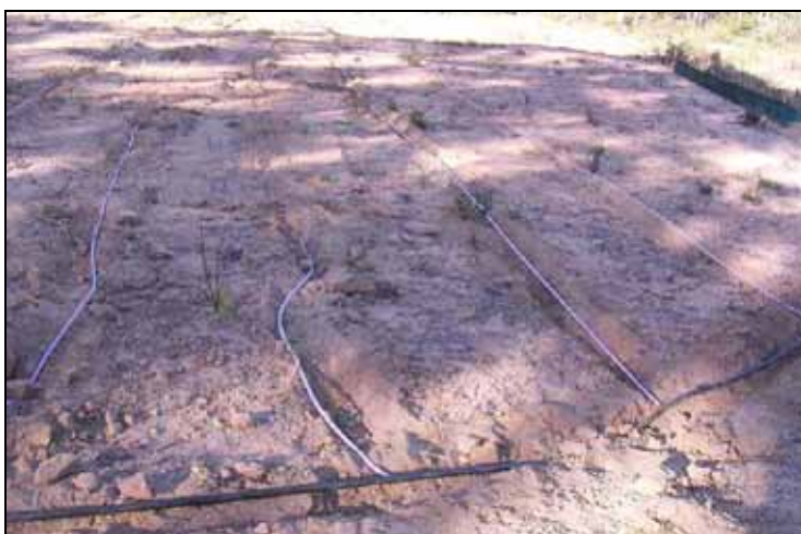
Figure 13.7 Poorly installed subsurface effluent irrigation system
