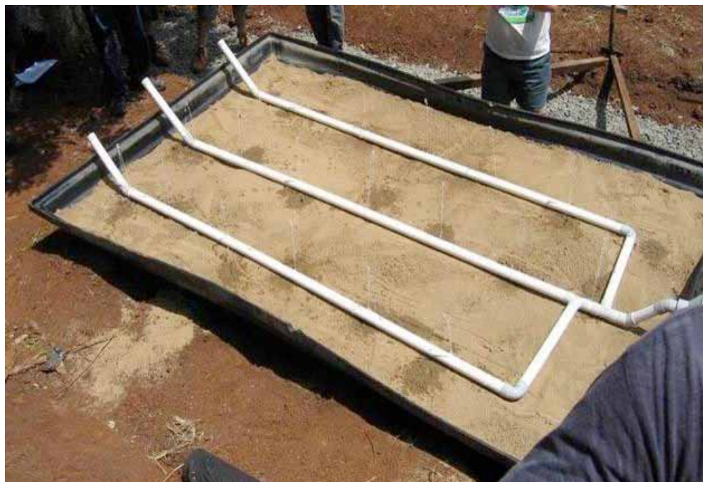
Figure 14.3 Siphon being tested delivering pressure dosed load to a sand filter (Inwater)
