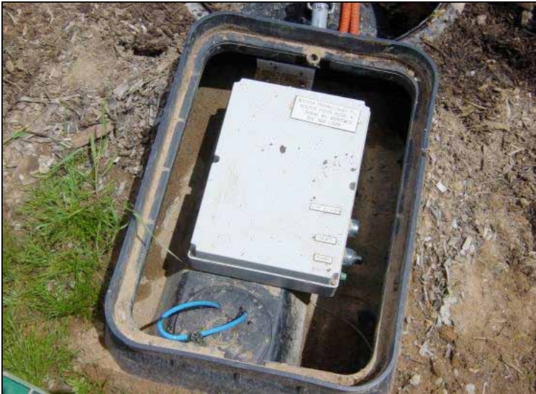
Figure 5.8 An electrical box that was flooded
