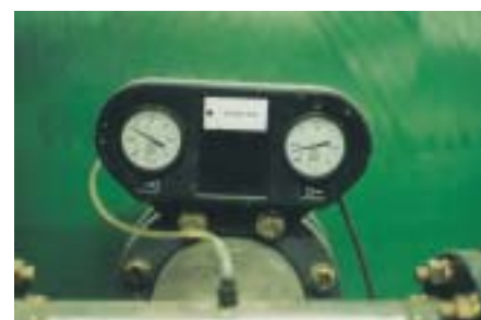
Figure 36 Pressure differential gauges
