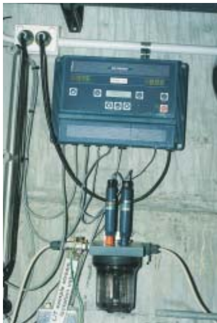
Figure 19 Chemical sensors installed in a side-stream loop
