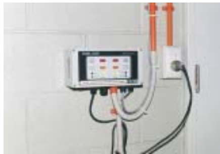
Figure 11 Ozone leak detector
