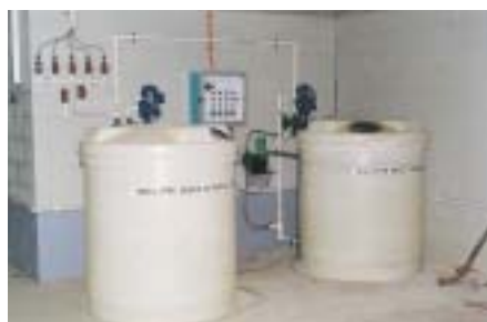
Figure 35 Dosing tanks with mixers for adding coagulant
