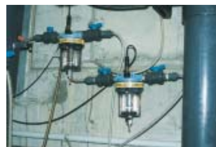
Figure 9 Pool water treatment with ozone and hypochlorite
