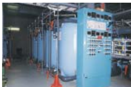
Figure 30 plant room with multiple filters
