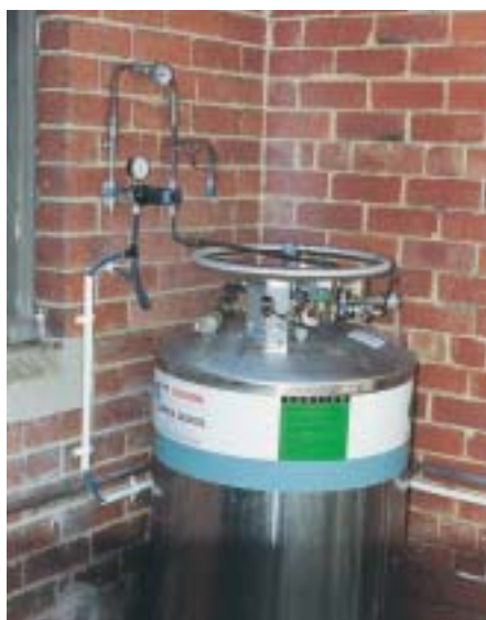
Figure 13 Carbon dioxide tank
