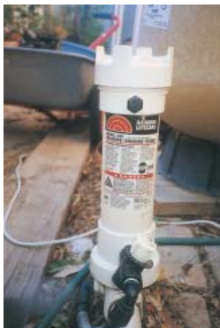
Figure 17 Erosion canister (erosion feeder)
